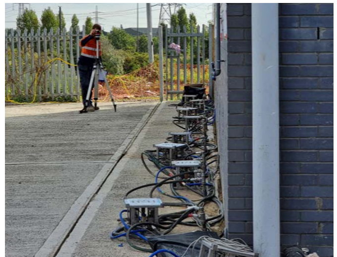
Above: A Mainmark technician checking building levels and the non-invasive JOG Computer-Controlled Grouting injectors placed around the exterior of one of the units.
