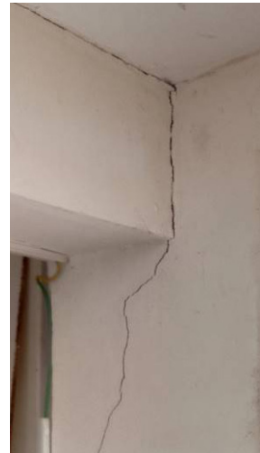
Crack on wall before treatment
