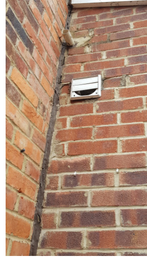
Visible gap where extension joined main house
