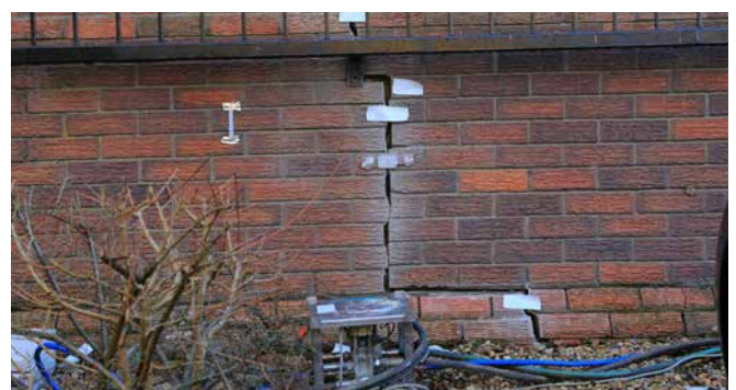
External wall cracks caused by subsidence
