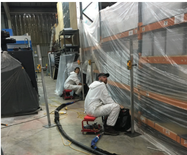
Mainmark Technicians injecting Teretek® engineered resin while monitoring the lift using a laser-receiver
