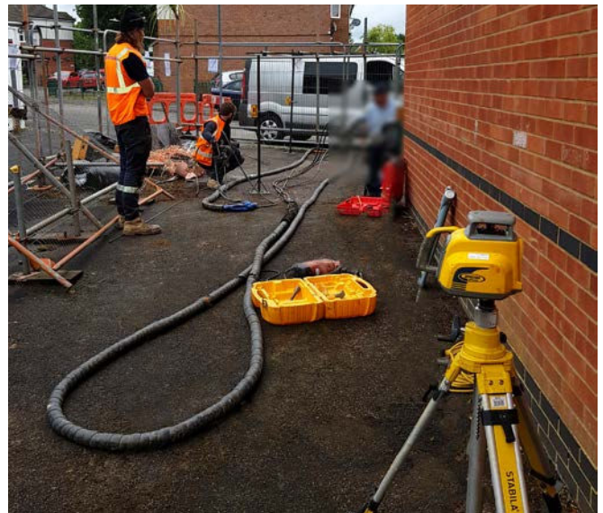
Teretek® resin being injected to fill the voiding and stabilise the top layers of ground in one of the designated areas on the property
