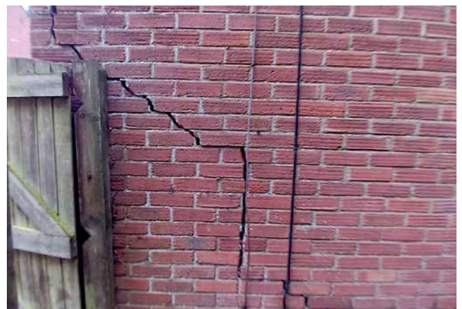
After Teretek® resin injection, the voids under the property were filled and significant ground improvement and lift were achieved, also helping to close some of the cracks
