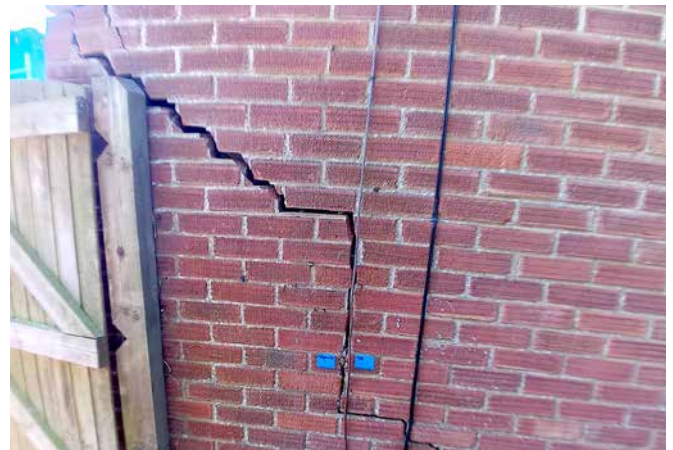
Cracking on external wall of the property before Teretek® resin injection
