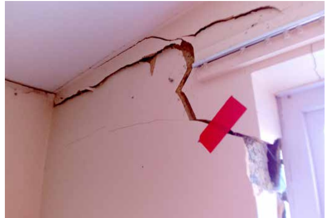
Significant cracking on wall of the property's ground floor
