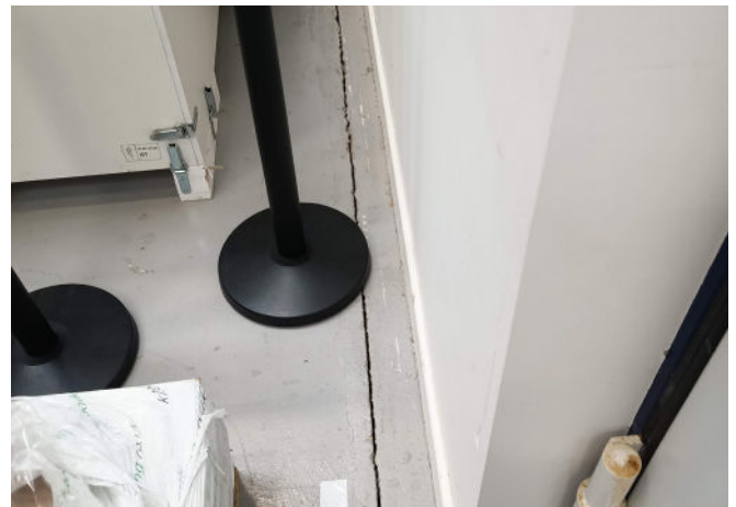
Concrete floor separating from wall caused by unstable ground and voids under concrete slabs
