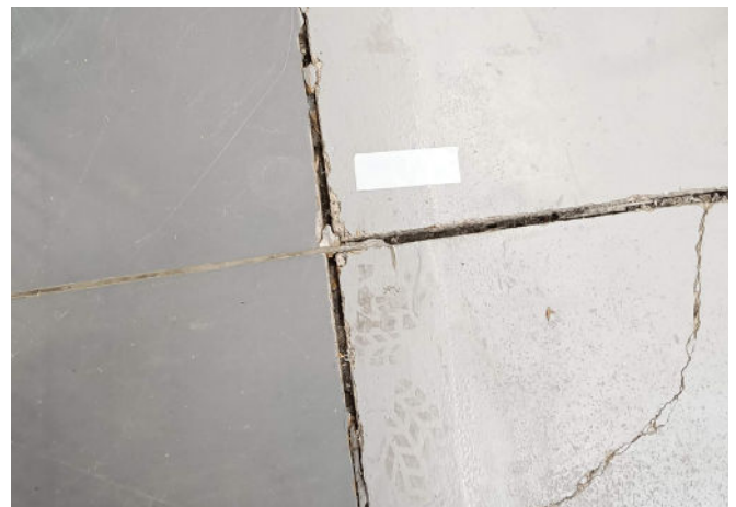
Severe cracking on laboratory floor
