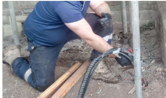
Teretek® material being injected into the work site despite scaffolding placed around the area
